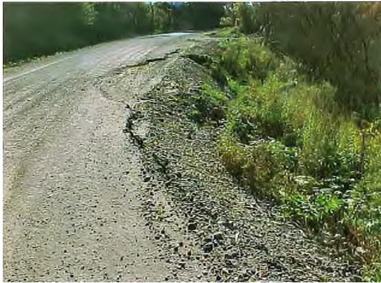
Figure 5.4.6-2. Landslide/Geologic Hazard in Town of Caneadea
